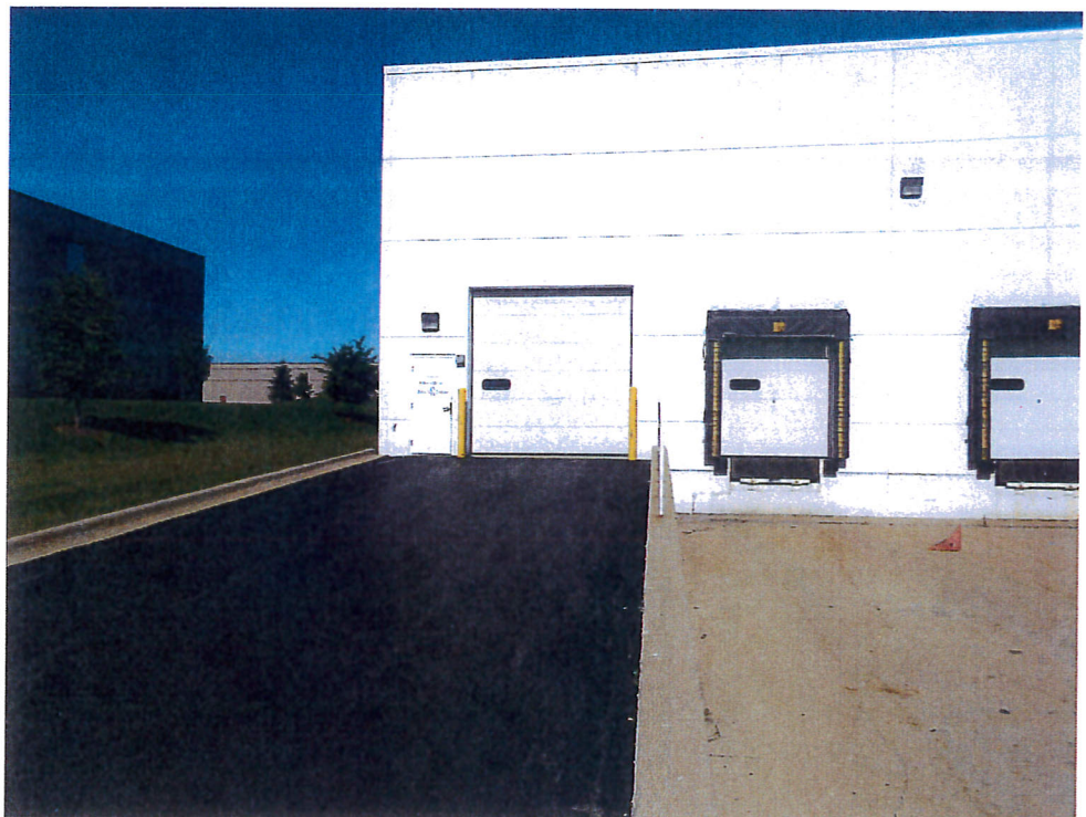
16) View looking west at the drive-in-door at the south end of the warehouse area. Note the retaining wall separating the depressed truck docks from the drive-in-door.
