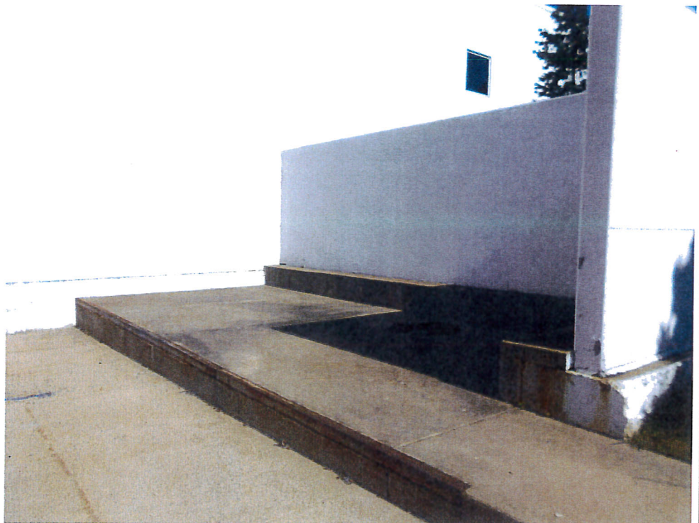
18) View looking north-west at the concrete "patio" area at the north edge of the depressed truck dock area.
